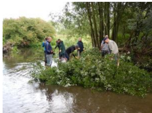
Swapping spreadsheets for wellies, some of the Environment Agency's SEP team hard at work building the willow deflector (Image © Mark Everard)
